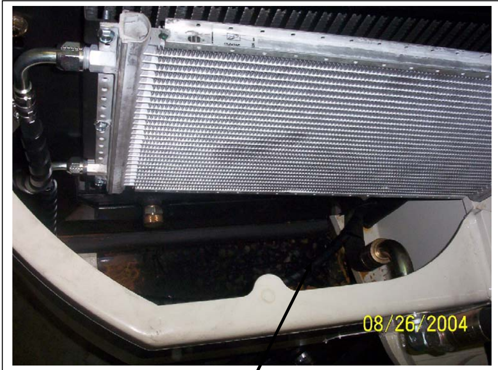
5/16" line from the lower fitting on the condenser running into the engine compartment area beside a hydraulic hose.
